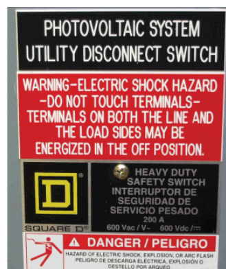
Plate 2. Label on PV disconnect
